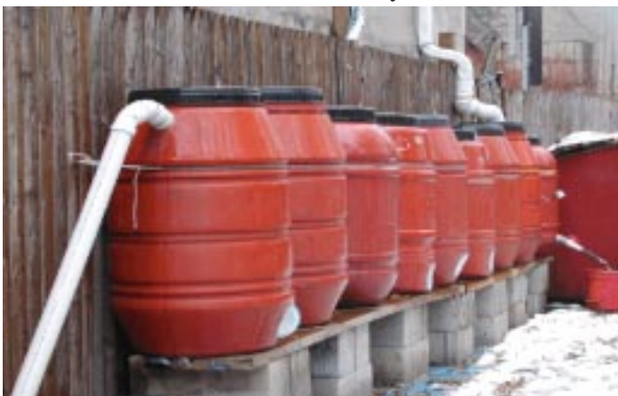
Rainwater Collection System at 1100 Bergen Street Community Garden in Brooklyn.
